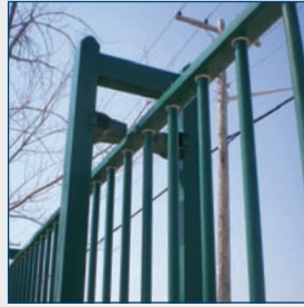
Portal and guide rollers
